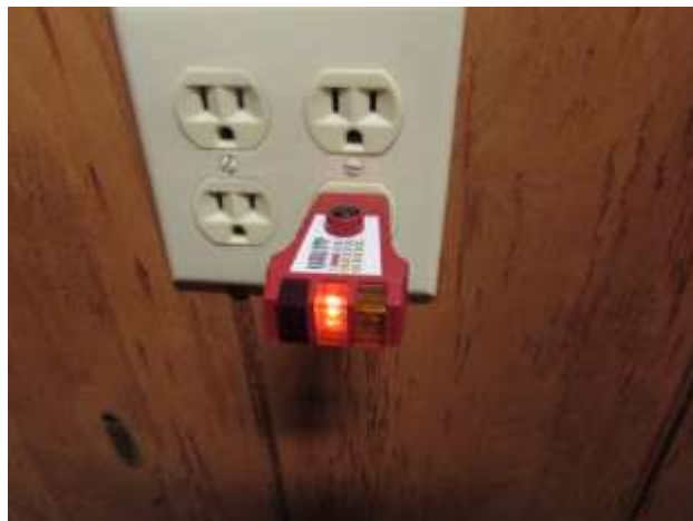
This dual outlet had the left side grounded and the right side not grounded.
