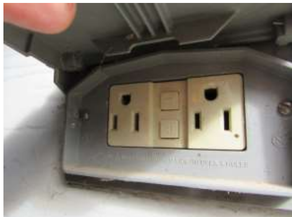
The GFCI mechanism did not trip in the west garage exterior outlet. Recommend replacing this GFCI outlet. Cycle GFCI trip mechanisms about monthly to keep them limbered up.
