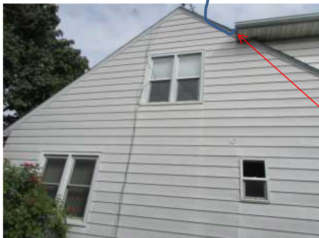
This hole is located right here. It is big enough for bats, though I saw no evidence of them. Recommend sealing this hole.
