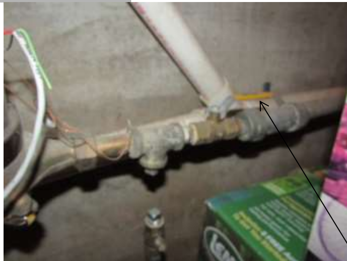
Main shutoff valve.
