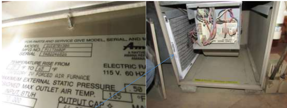
Note filter location.
